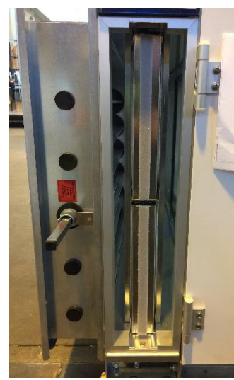
Figur 140: borttagen Dörrpanel (TRA)
